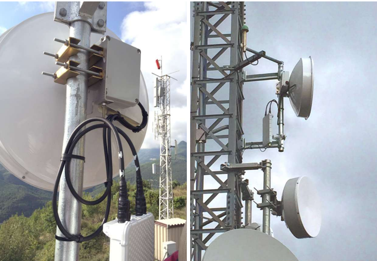
The picture above is one side of the link installed in a Serra di San Quirico municipality
